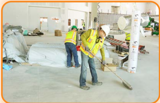
Thoroughly sweep the surface to ensure the area is clean and free of debris/foreign materials that will compromise and contaminate the Base Coat.
