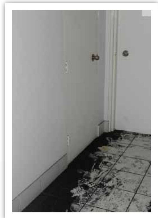
Unprotected tile required replacement after fire and smoke damage
